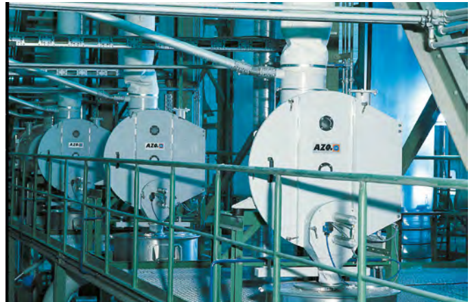
AZO®MIXOMAT mixers above processing machines
